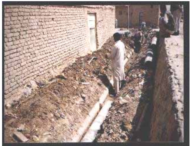
Construction work of laying a sewerage line in progress in one of the Katchi Abadies of Quetta
