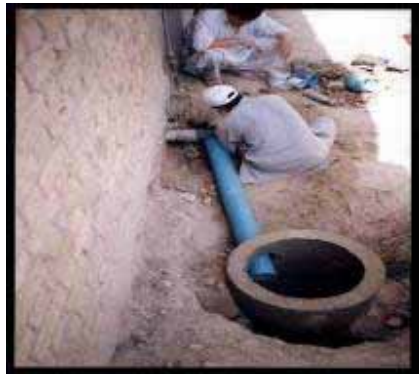
Masons are busy connecting P.V.C. pipes from a house to Tee Hodi in a lane at Hazara Town, Quetta
