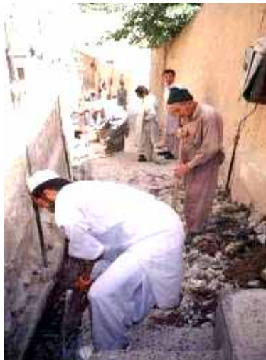
Masons and labourers are carrying out construction of sewerage line. The Engineer and Social Organizer (in the background) are supervising the work
