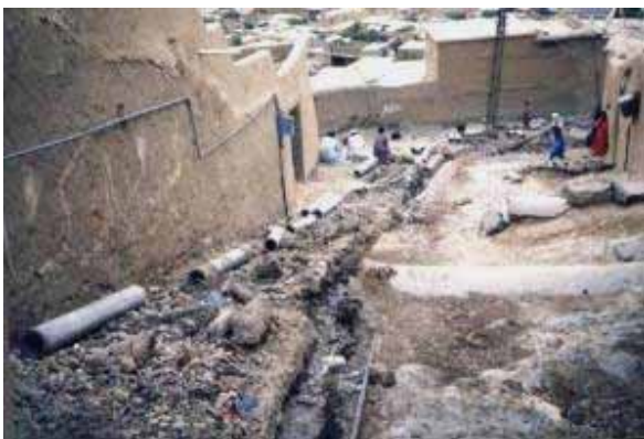
9 inch pipes being laid to cover the open drain in one of the lanes in a Katchi Abadi
