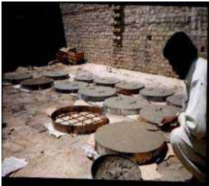
Manhole covers reinforced with steel bars and G.I. sheet rings being constructed near the construction site
